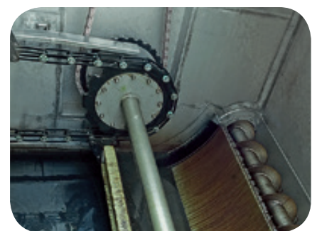
Sludge removal using of screw conveyors
