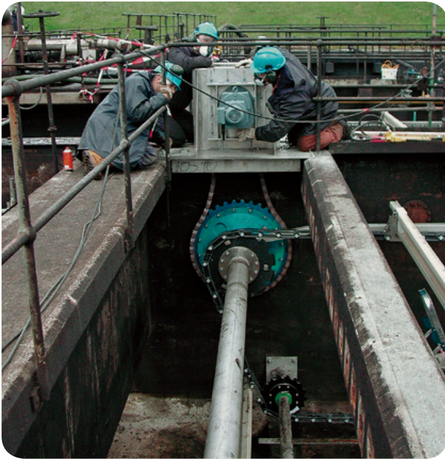
API sedimentation tank in the refinery
