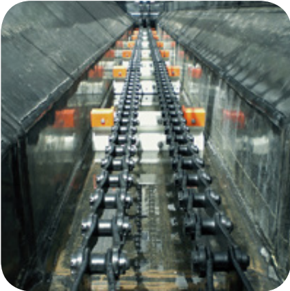
Grit collector scrapers
