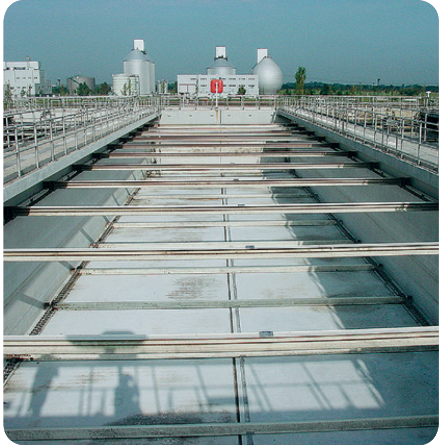
Bottom sludge and floating scum scrapers
