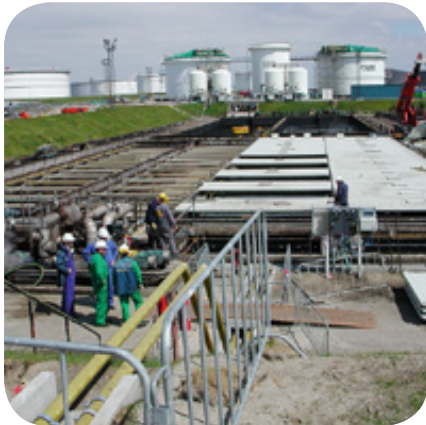
Refinery, the Netherlands
