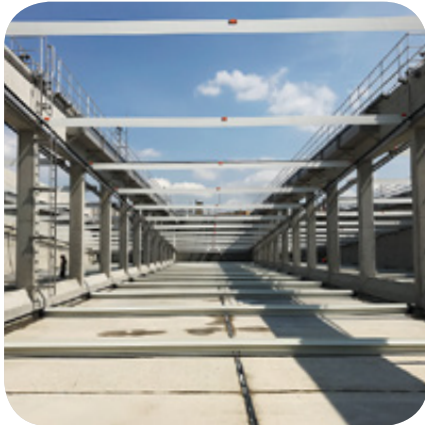
Bottom sludge and floating scum scrapers
