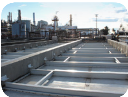
API tanks with floating covers
