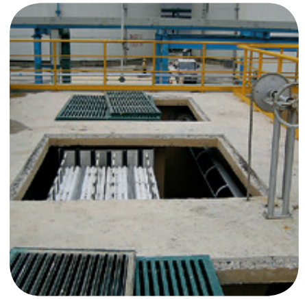
CPI installations with covers
