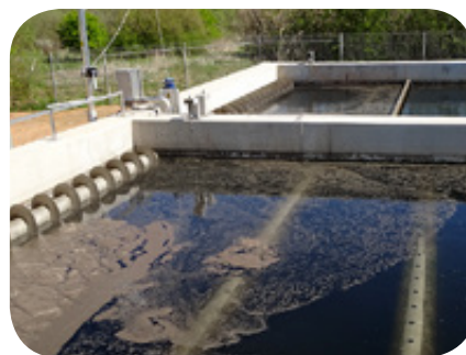
Rectangular tanks with submerged drain tubes and screw conveyors for floating scum removal
