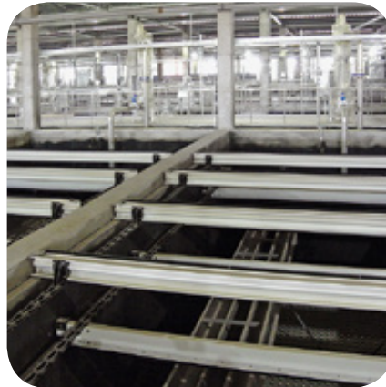
Drinking water treatment, Kazakhstan
