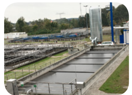
Municipal waste water treatment plant with chain scrapers
