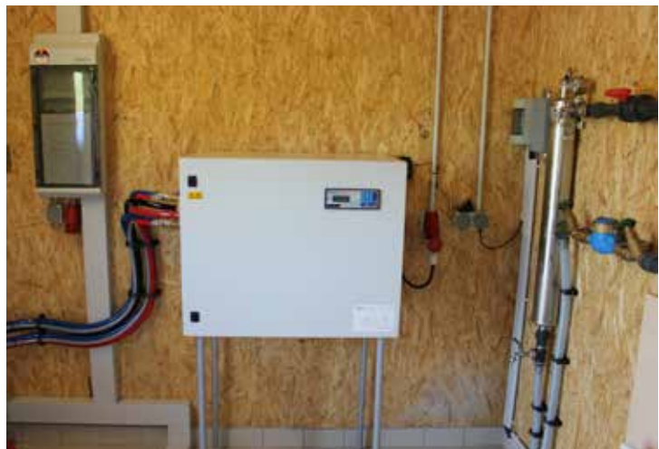
Power distribution board, switch cabinet, UV module
